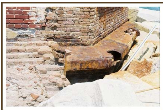
Damage to Cast Iron Ring on West Side of the Base of the Lighthouse
